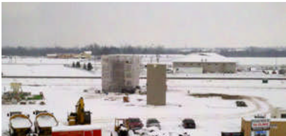
The temporary shelter pictured above encloses the stairwell for the soon to come Ramsey, Minn. facility.
