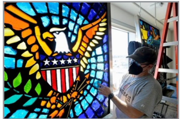
A stained glass window that formerly hung in the Lincoln Community—Based Outpatient Clinic (CBOC) chapel is reinstalled into the new Lincoln Super CBOC in March as a part of a display honoring the heritage of the former VA hospital and CBOC that had been in operation since 1930. (Photo by Kevin Hynes)
